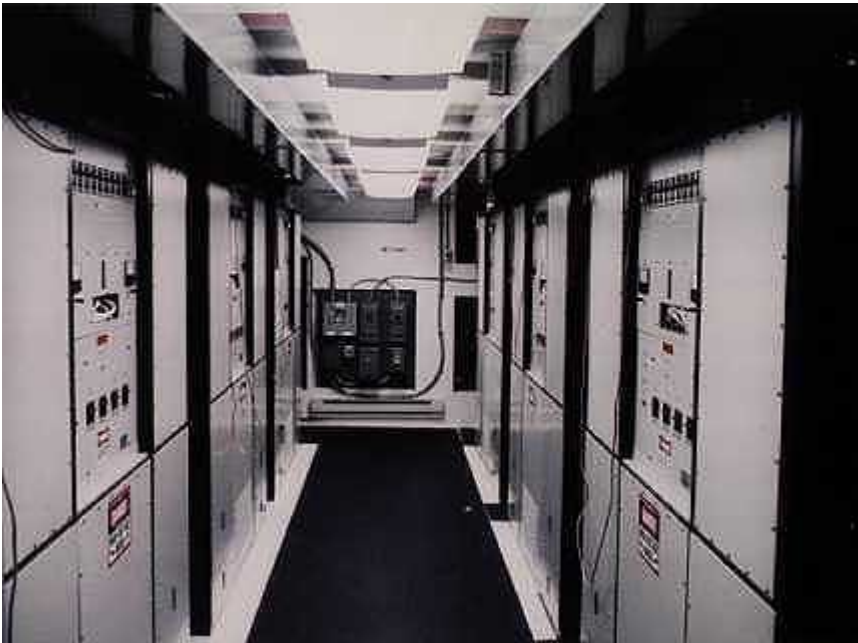
Image 4: Inside the Transmitter Shelter
